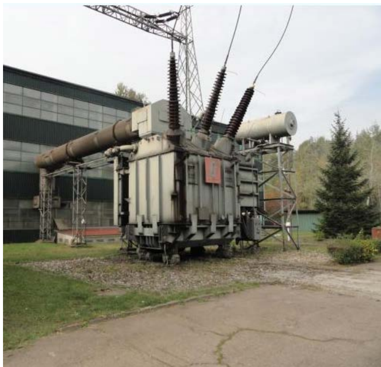
Step-down Transformer (Photo by Zurich RE Pat Dunphy – 20131022)
